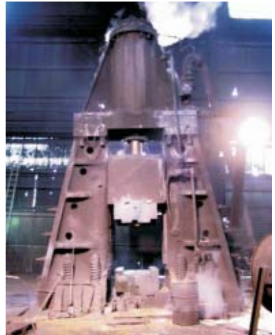
Before the revamp, foundation failure caused Kropp Forge's Erie steam hammer to tilt to the left and front.
