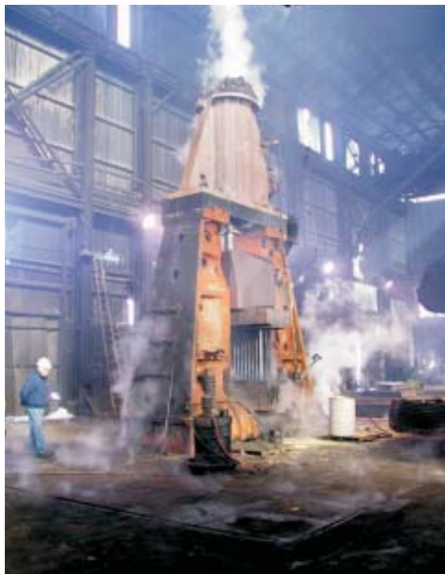
Erie 50,000-lb steam hammer ready to operate after installation of Vibro/Dynamics MRM Isolation Elements.
