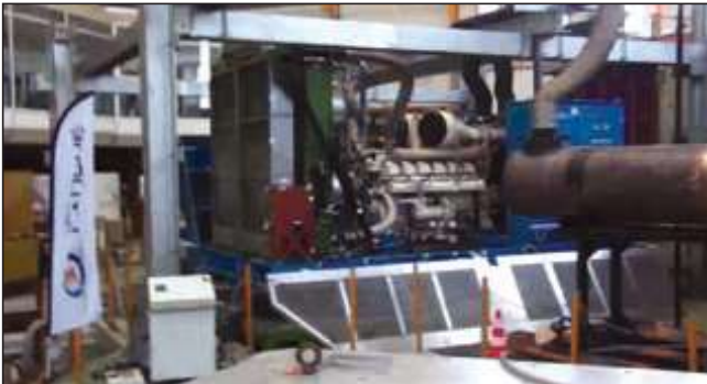
Figure 12. Physical test setup of genset.
